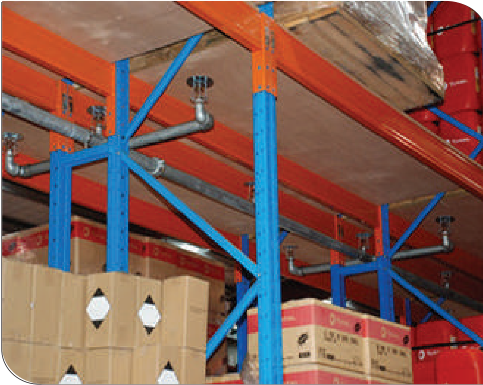
In-rack Sprinkler System
